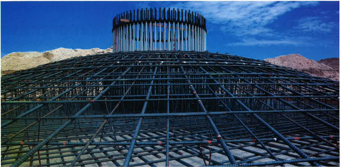
The white cylindrical flanges will be bolted to the tower section before the turbine components arrive.
